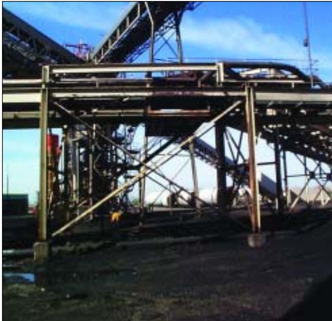
Conveyors are often subject to aggressive, exterior exposures.
